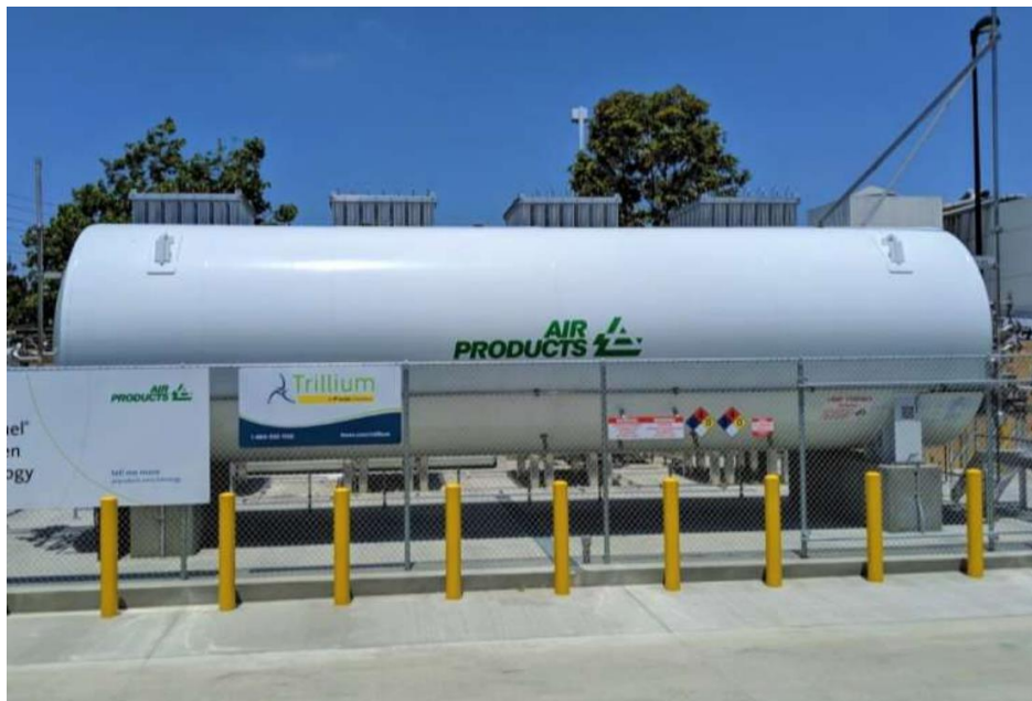
Figure 3-2. OCTA Hydrogen Tank
