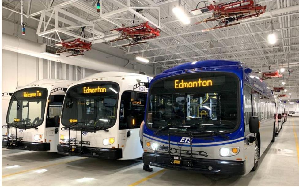
Figure 2-4. Bus Operating Facility, Overhead Pantograph Chargers, Edmonton Transit
